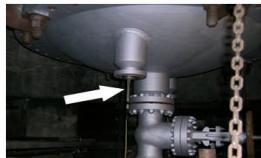
5. Thermocouples crossing process connection
